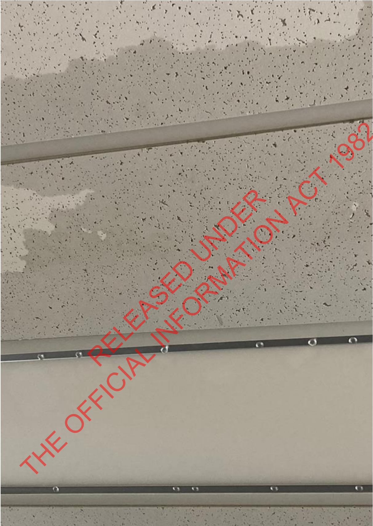
Photo 3: Water damage to ceiling tile and light fitting.
