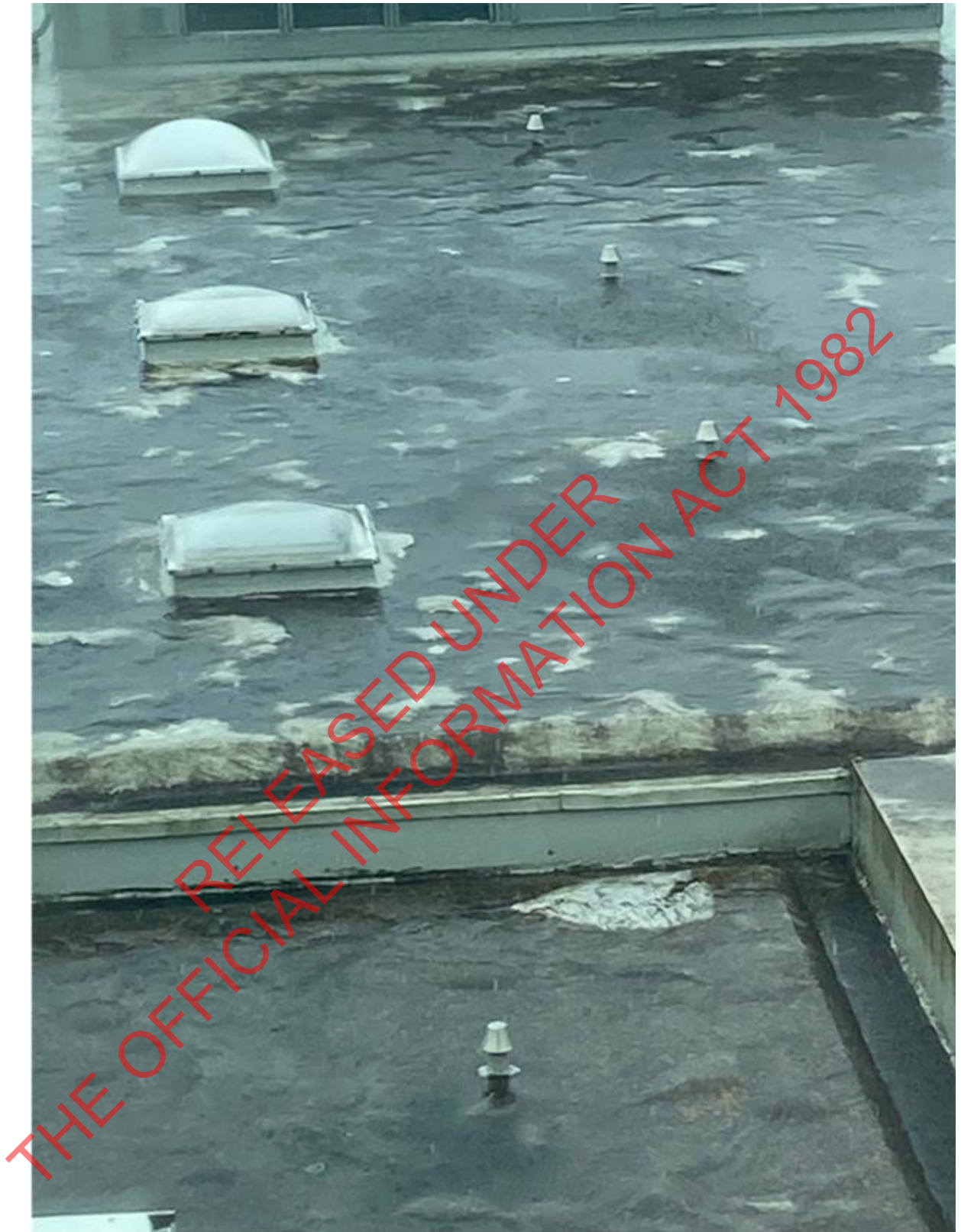
Photo 2: Close-up showing 'lunar landscape' and pooling in low areas of the roof.
