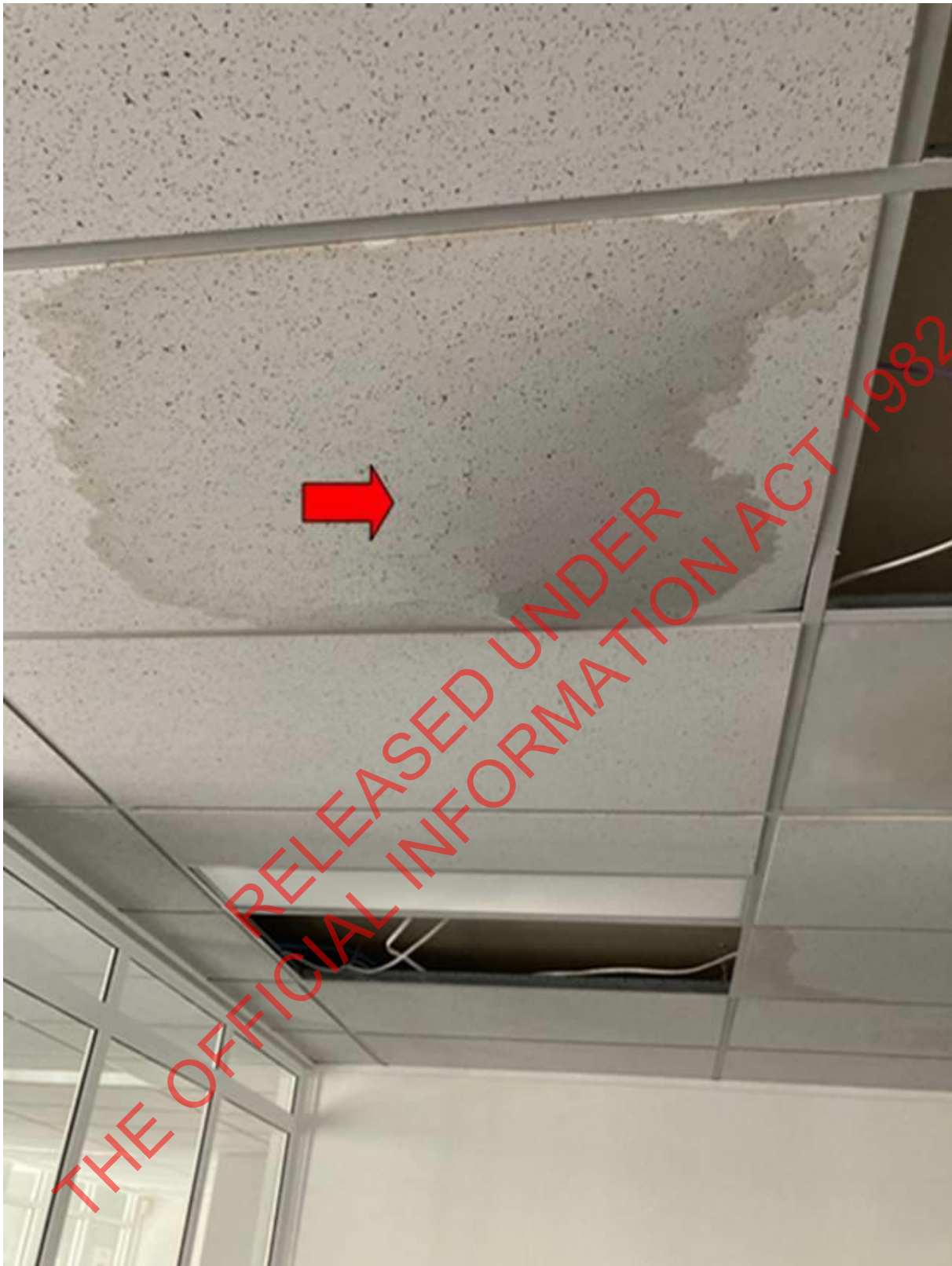
Photo 5: Showing ceiling tile sagging under the weight of the water absorbed into the tile, moments before it collapsed completely over the check-in area of the terminal
