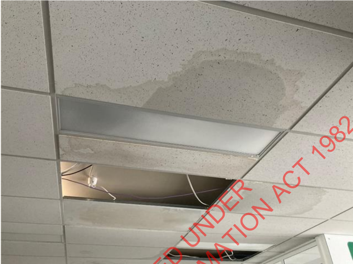
Photo 4: Water damage to ceiling tiles and light fitting and heater fitting.
