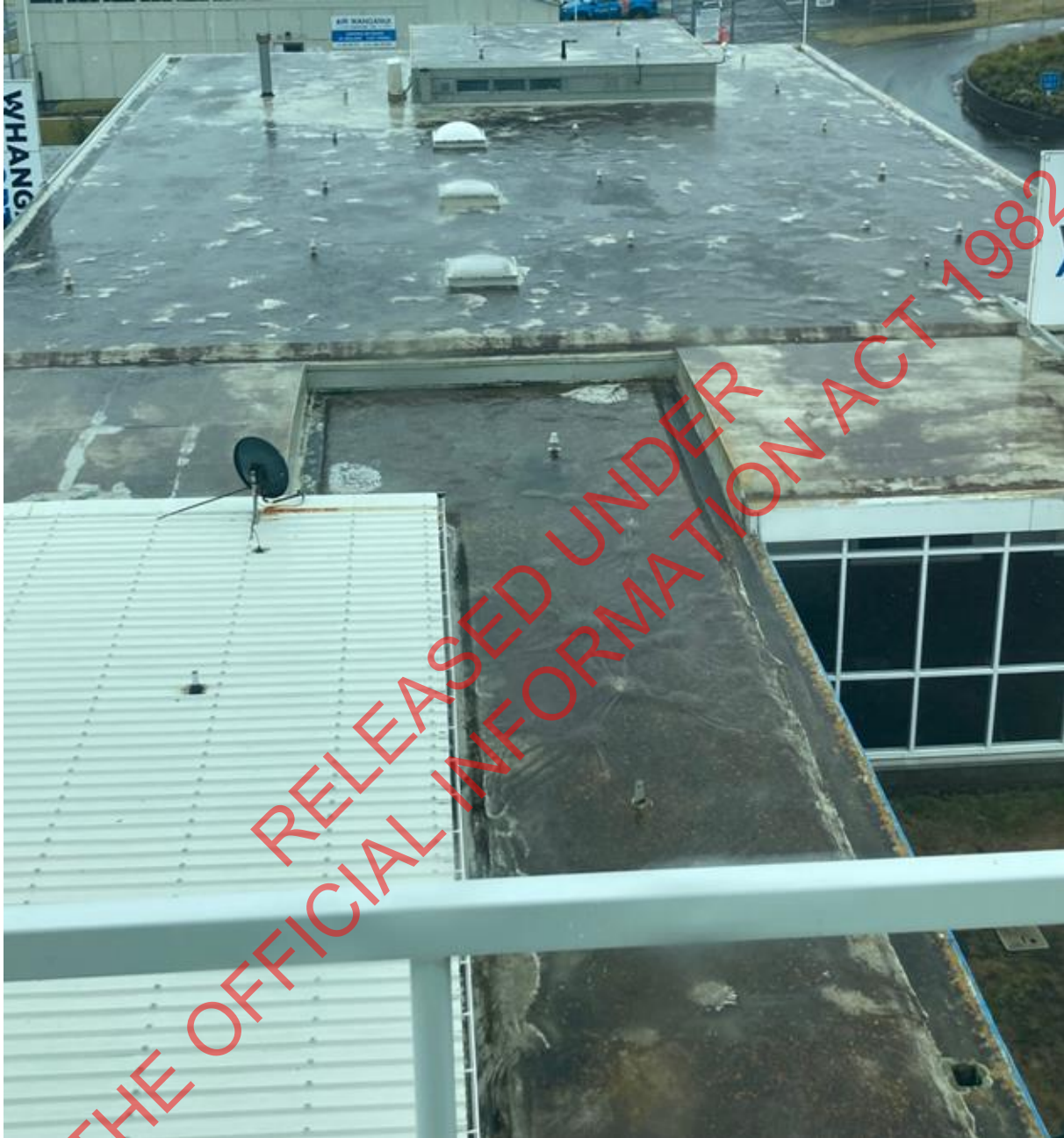
Photo 1: Overall roof image. Foreground shows bubbles formed by original membrane deteriorating and damaging top layer. Internal gutters rarely dry out due to design of roof and minimal 'fall'.
